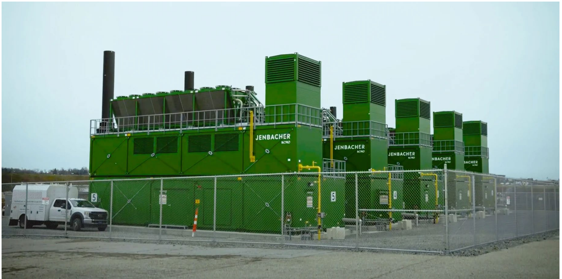
Comparable facility with containerized Jenbacher engines.
