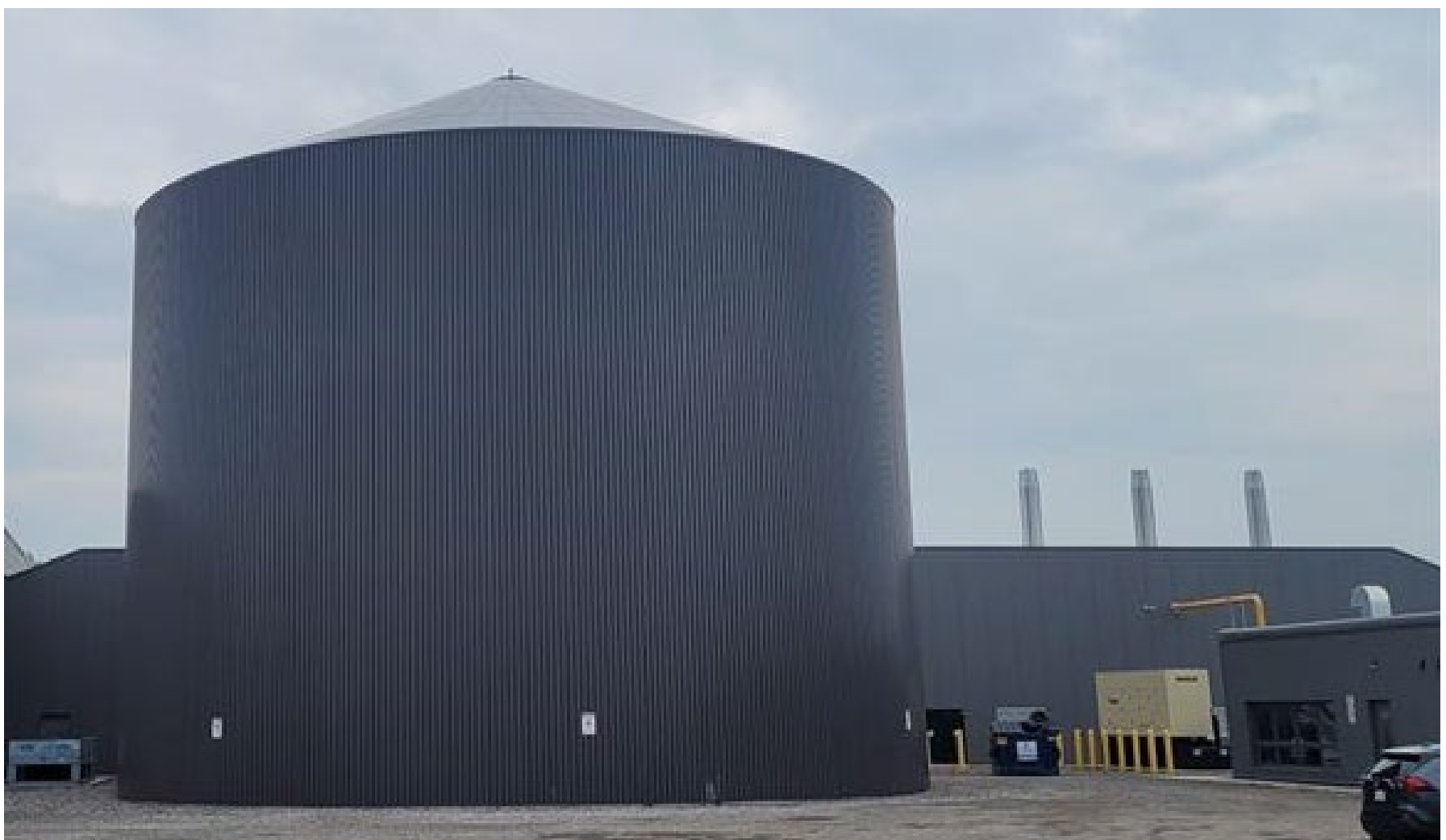
Heat storage tank at a comparable facility.
